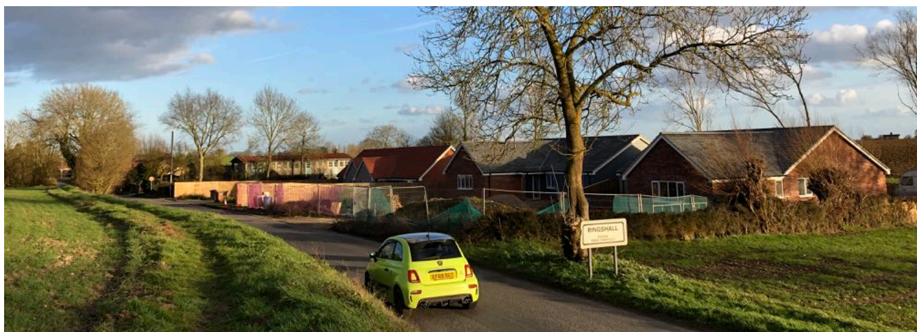
Ringshall Stocks approaching from the west on Lower Farm road. The two new bungalows 1 & 2 'The Willows' on the end of the village nearing completion.
